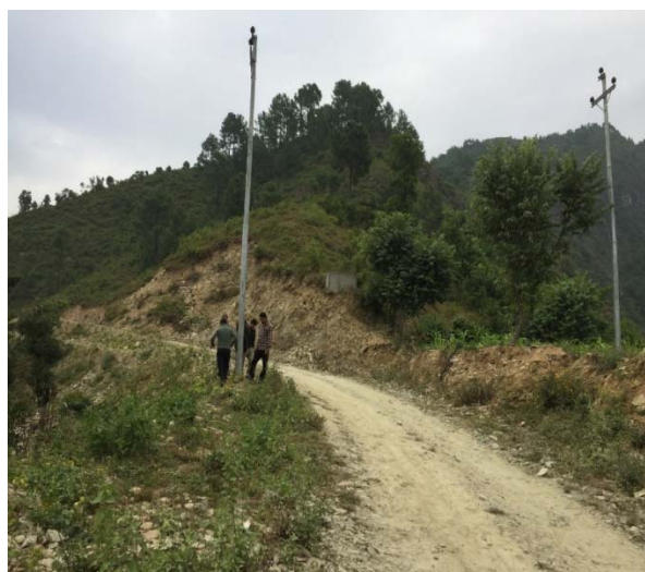
Pic 1: 11 kV line passing over the road in Bhirpani Village, Ramechhap district
