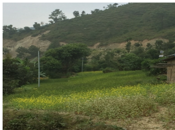
Pic 2: Poles installed at the edges/bonds of land in Bhirpani, Ramechhap district
